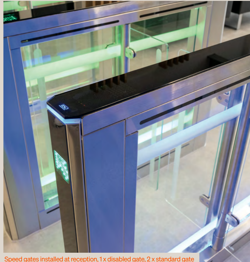
Speed gates installed at reception, 1 x disabled gate, 2 x standard gate
