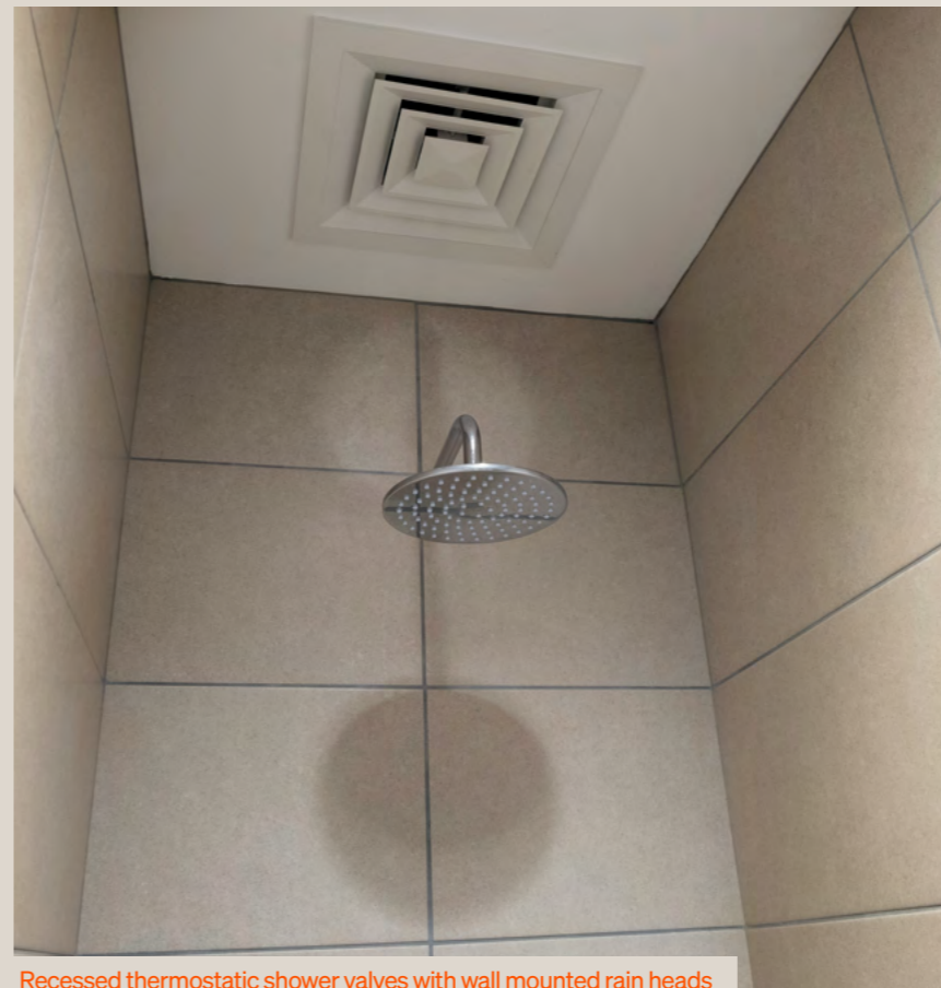
Recessed thermostatic shower valves with wall mounted rain heads
